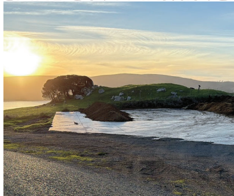
Straus Dairy Farm was awarded a grant that paid for a concrete composting pad to support a multi wind row composting system.
